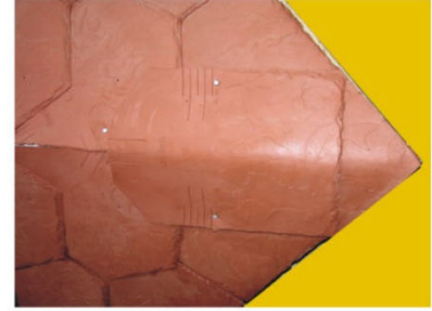
Picture 3: Install the next shingle as shown above. Additional nails may be used to firmly secure shingles. Repeat this step until you reach the top.
